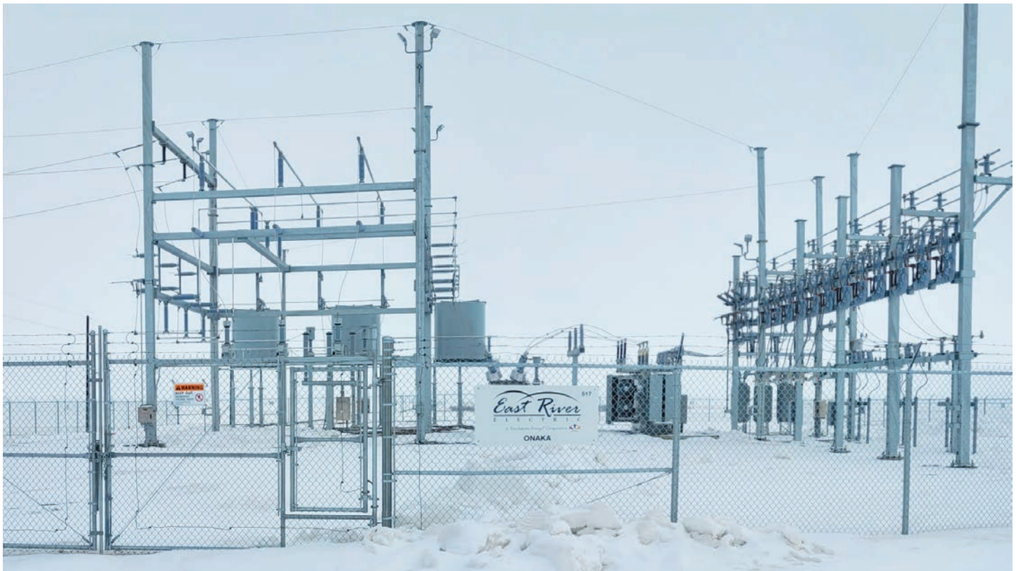
Bottom: The new Onaka substation powered by East River Electric.
