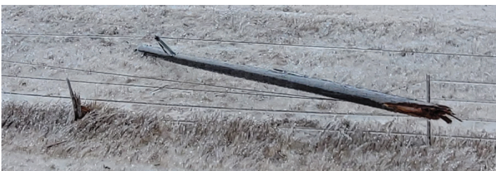
Below: A broken pole from the Christmas ice storm.
