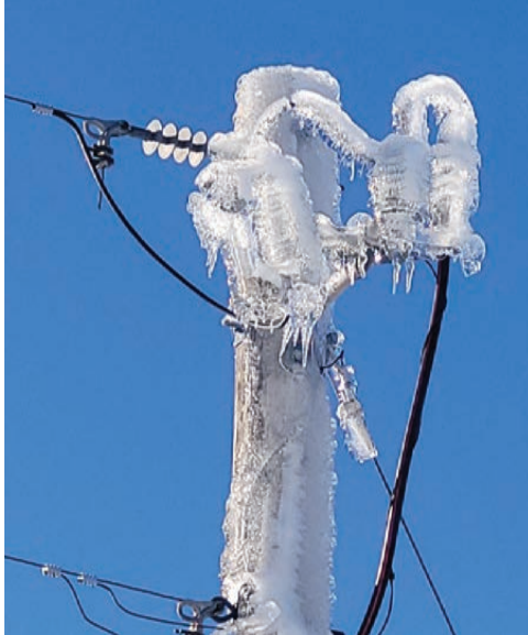
Above: Over an inch of ice coats equipment from the Christmas ice storm.
