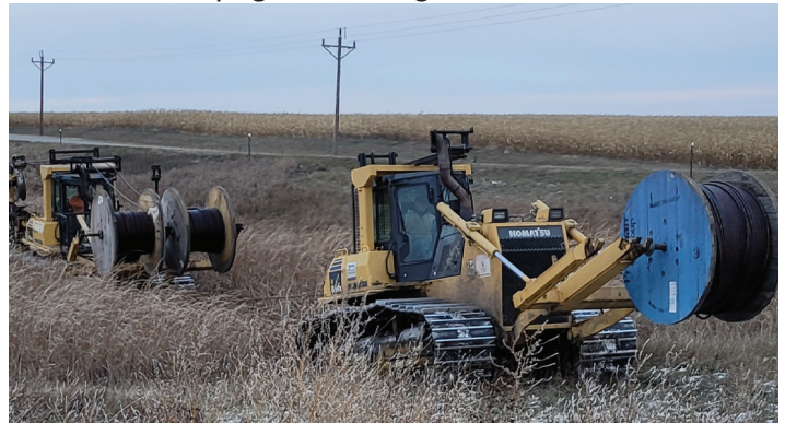
Below: FEM crews work with K&H Construction, replacing old line and burying new underground line.
