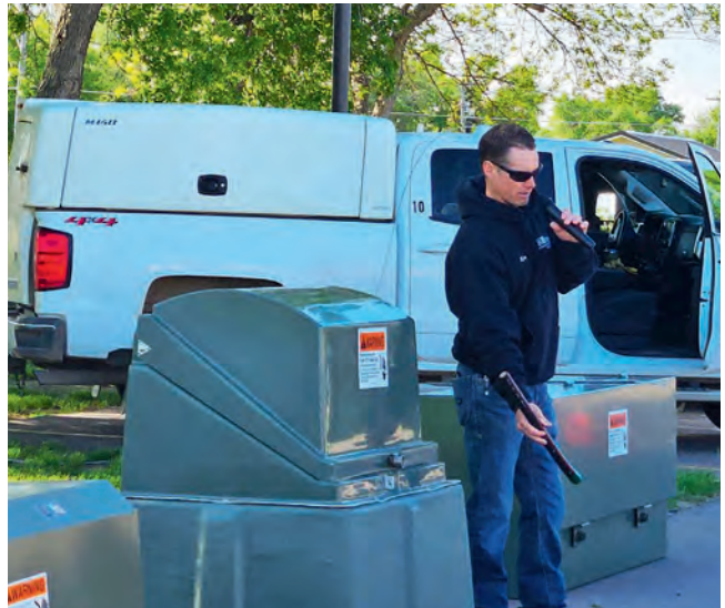
Ryan demonstrates how underground wire comes into an underground cabinet. He warns kids to not play on them as there are thousands of volts of electricity running through these cabinets.
