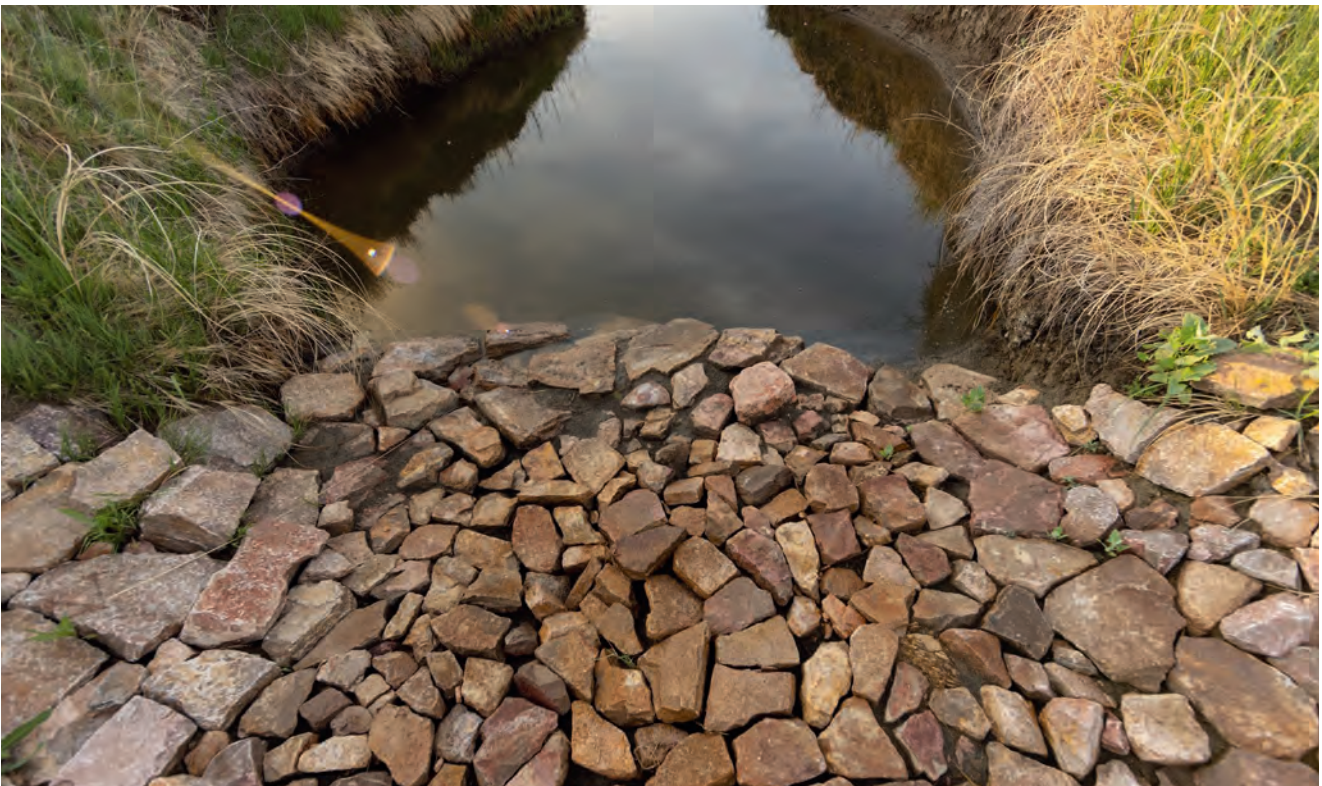
A rock structure installed to help prevent headcuts from eroding upstream reaches. Photo Credit: Joe Dickie, Generation Photography, Inc.
