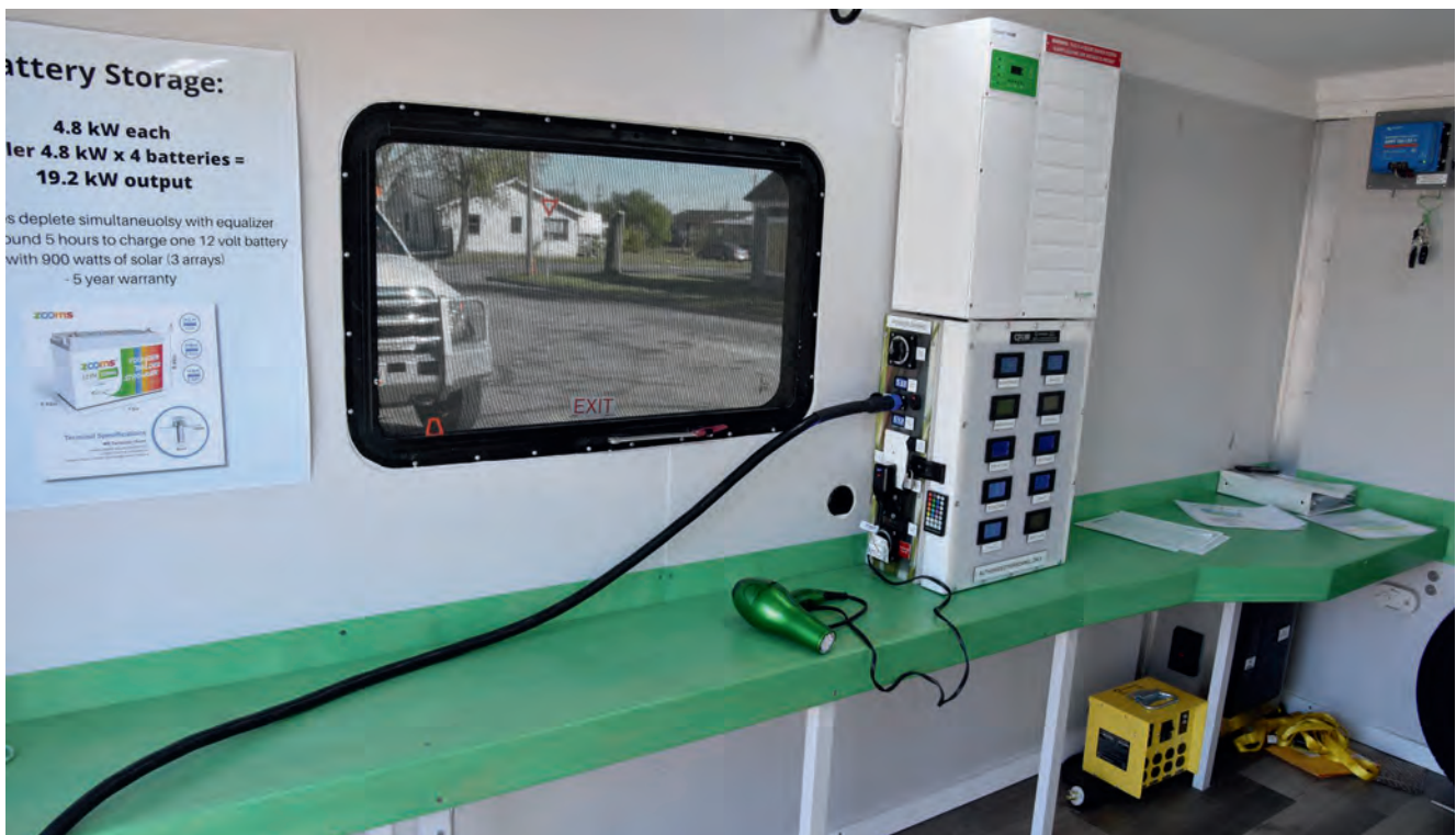
The interior of the solar trailer is equipped with battery storage and outlets – powering everyday electrical appliances, such as a hairdryer.
